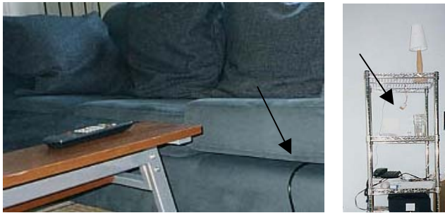
Figure 1: A pressure sensor installed on the TV sofa (left) and an infrared sensor hung on a shelf near the desk (right)
